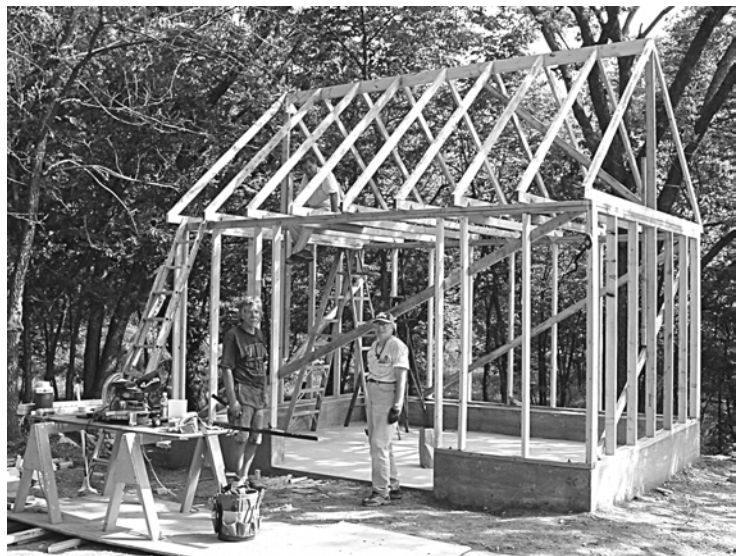
The frame of the new shed at HH with Sue, Jan O. and Charlie.
